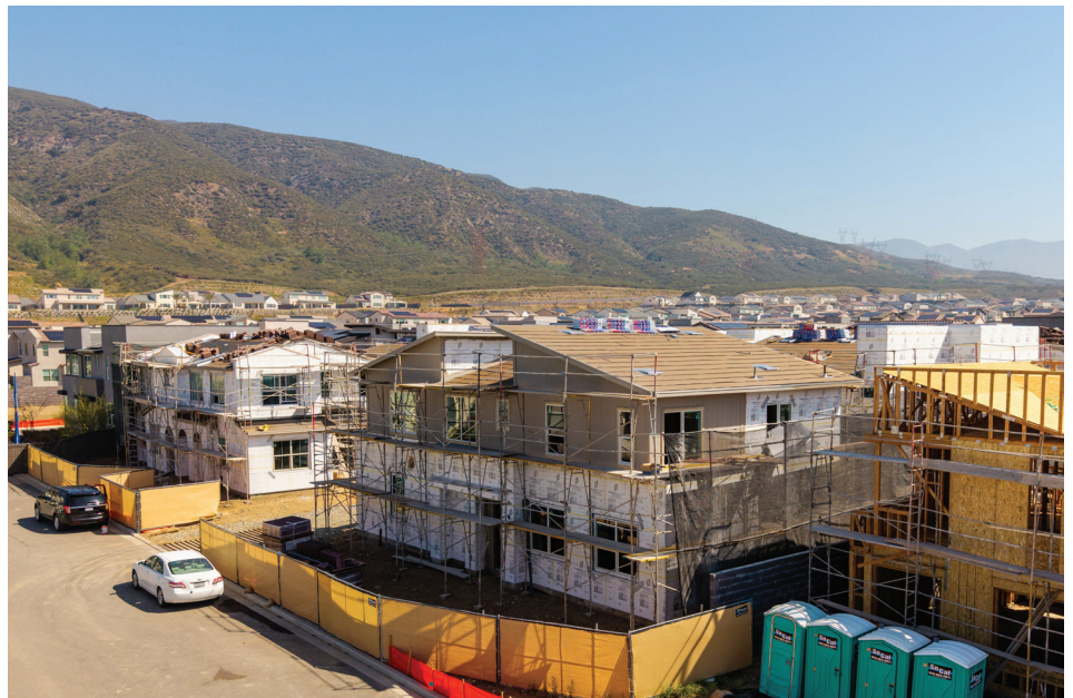
Homes under construction at a development in Fontana, California. Photographer: Kyle Grillot/Bloomberg
