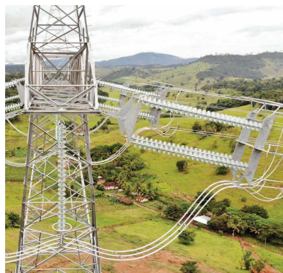
Sediver glass electrical insulators
